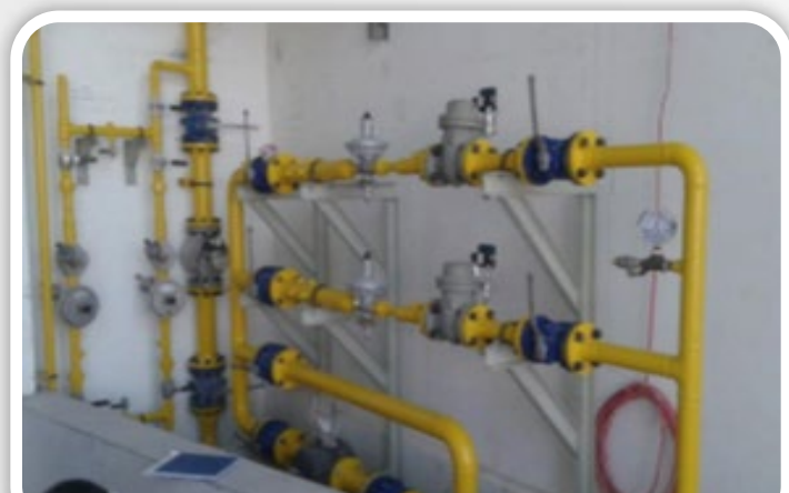
Pressure reducing station (SNG system) at Sigma 2
